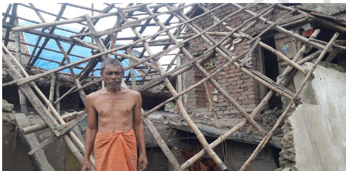
House Damage due to “AMPHAN” Khejuri-II Block
